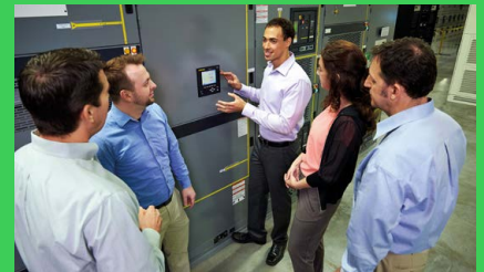
Growth through reliable operations supported by EcoStruxure™
